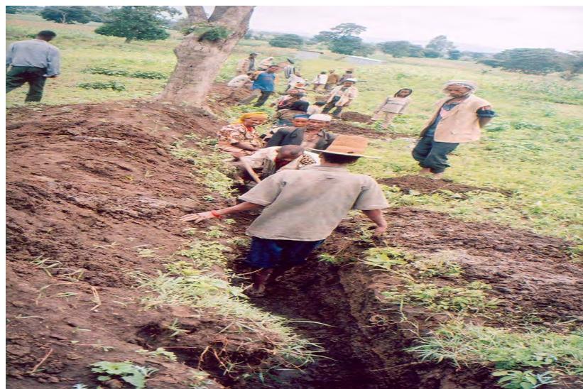
Water supply pipe trench excavation through community donated labour in Simbita Kebele
