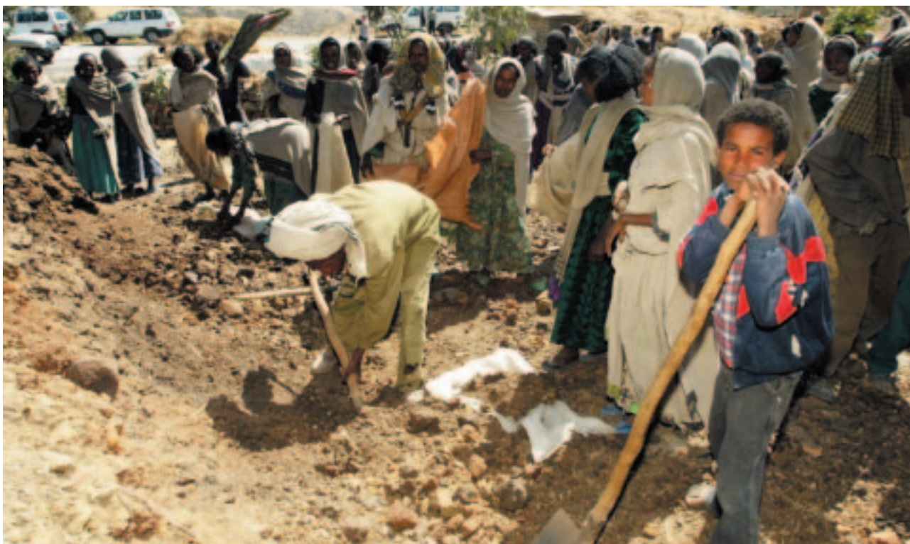
Men and Women working on a road building project in Northern Tigray, Ethiopia. Courtesy: Ó Maxwells
